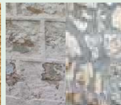
Joint en saillie Joints ciments
